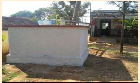
Picture (2.2) Water harvesting tank halfway above ground
