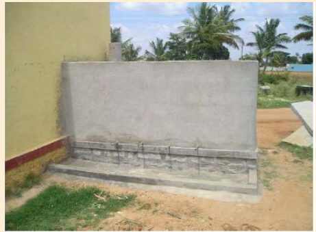
Picture (2.4) Water taps outlet system and cemented area below the tap for letting wastewater disposal
