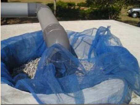
Picture (2.1) Filter at the entrance of tank
