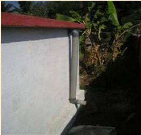
Picture (2.3) Overflow pipe with mesh
