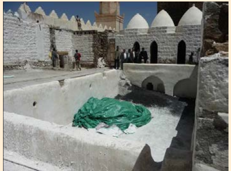
Picture (8.5b) Roof rainwater harvesting from a Mosque roof to mousque pond in Jiblah, Yemen (poho: sharaf 2011)
